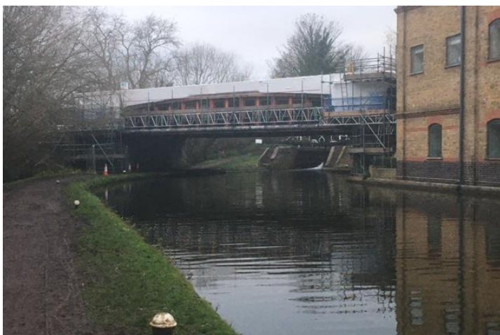
We hope to make this bridge look as good as the Ravens Lane bridge
